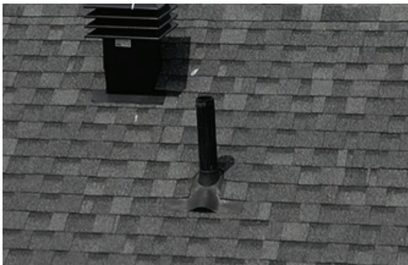
Example of (uncapped) radon pipe through the roof.
