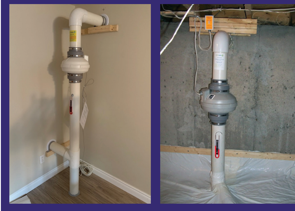
Examples of what an active depressurization system may look like in your home.
